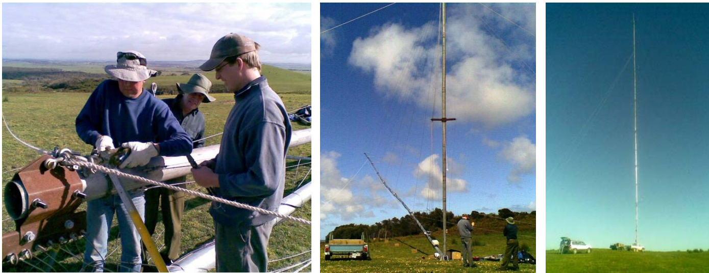
Data Tower Installation. A combined effort of Enviromet, Wind Power and a local land owner saw the recent erection of a 60m data tower.
